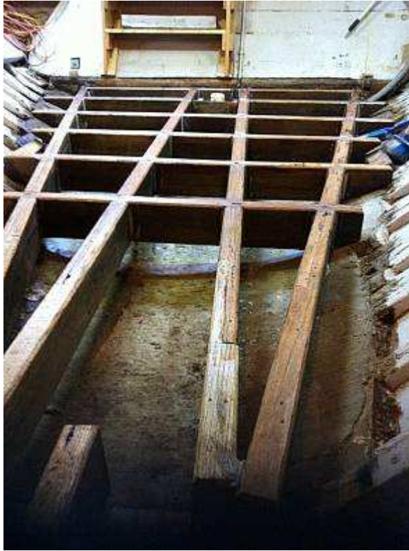
New sub-floor bearers were installed to support a new floor. The original 1915 layer of concrete on the hull was in good order.
