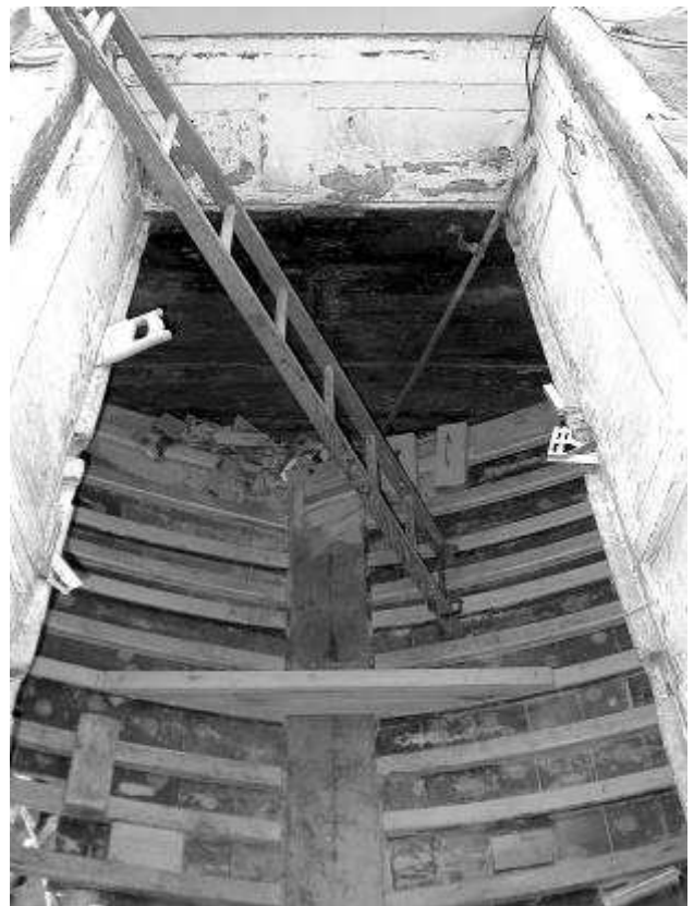
Fig. 4. The new keel top and all the new ribs are in place. One of the new floor timbers is in place. Seven new floor timbers were installed, fixed with 30 cm long copper dums through the floors into the keel.
